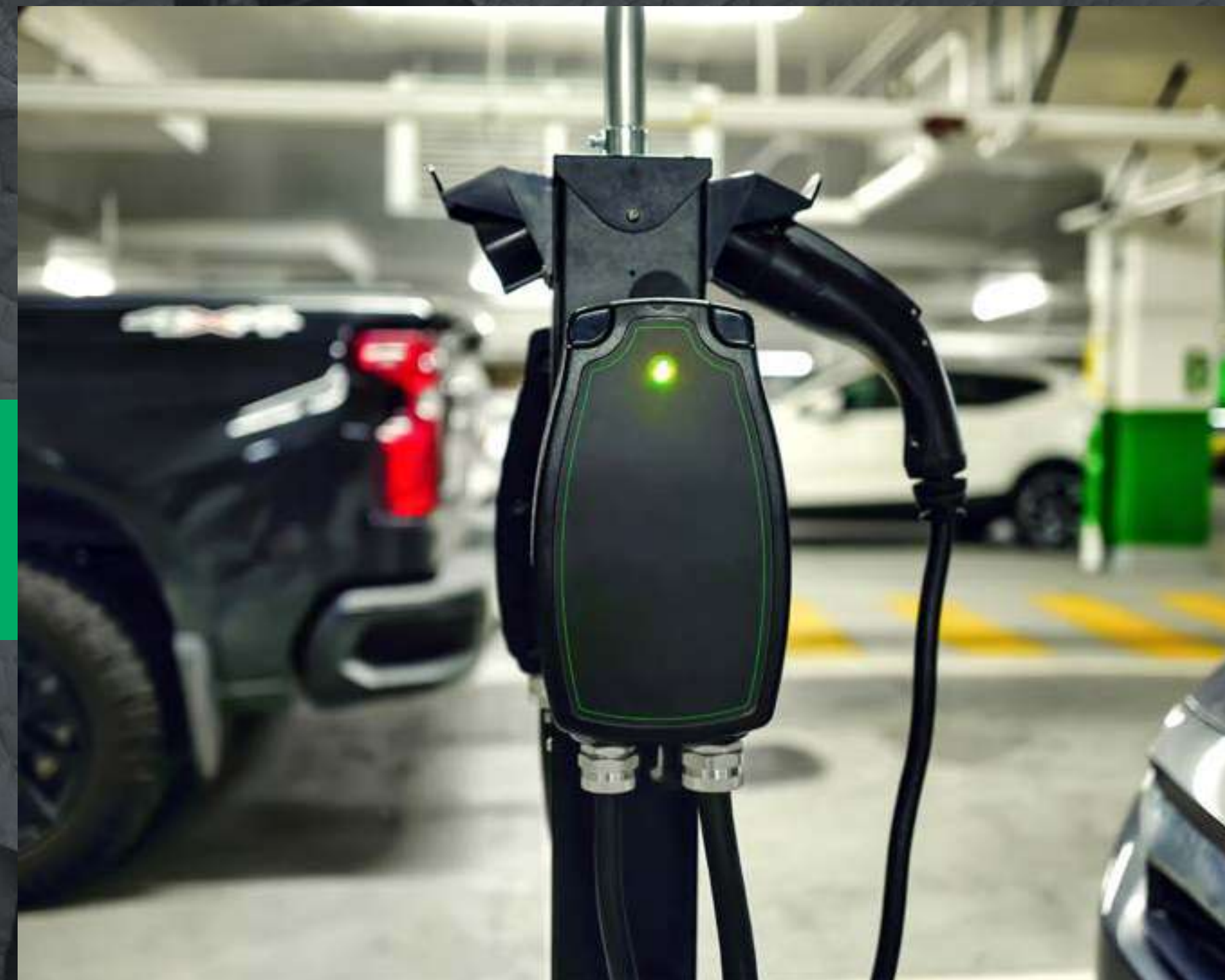
Electrical charging station in shopping mall
